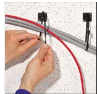
Without additional effort only Q-ties can be used for temporary and final cable bundling.
