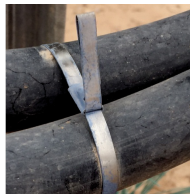
Protective coat is gone, exposing the metal parts.
