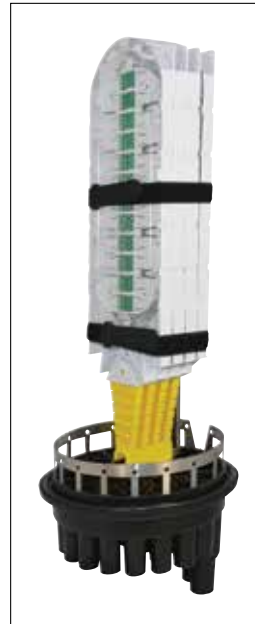
UFC C-length Closure with Hellamass Trays
